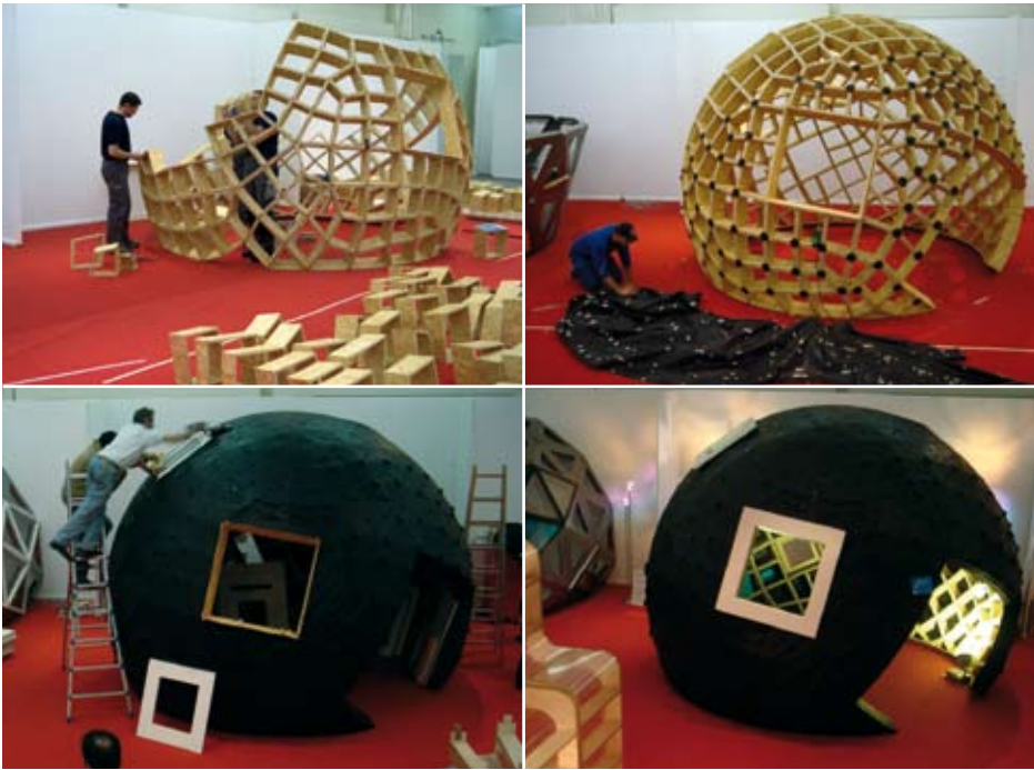
Assembly on site only takes a few hours. The quadrilateral frames of the wooden construction are prefabricated. They are stacked on top of each other like in a brick construction and connected by screws. The roof membrane is delivered in two large pieces and connected on site. Finally the windows are set in.
