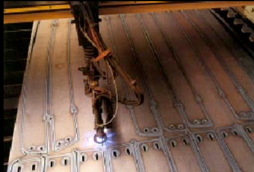
Plasma-arc CNC cutting of steel supports for FOG+Assoc „Zollhoff Towers“ in Dusseldorf
