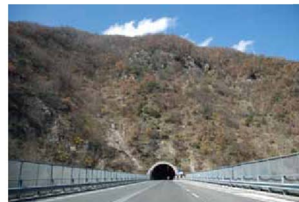
The Road mostly is elevated in a similar way of bridge, and carved into the mountains.
