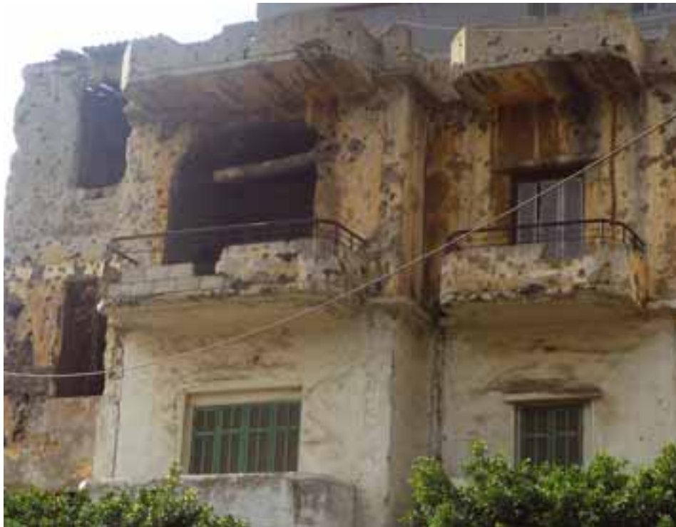
left: one of the houses in the very south of Badaro right: temporary use of a damaged building
