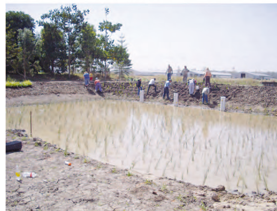
One of the managing activities: Construction and planting of a wetland to restore the lost wetland amount
