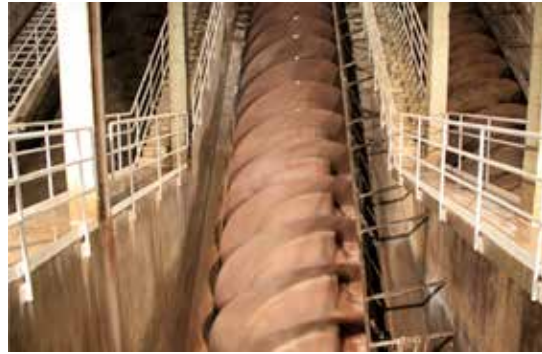
ARA Pro Rheno Basel/1. Pumping Process
