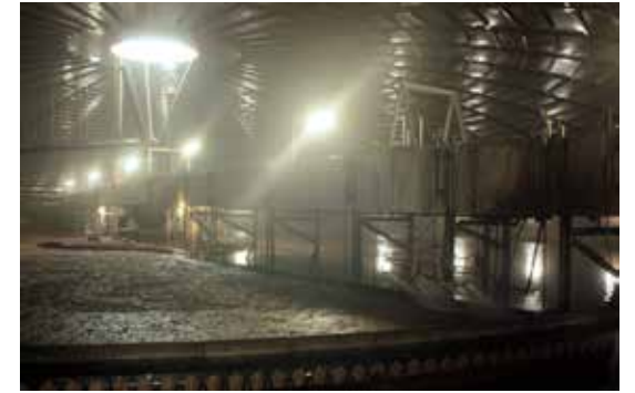
ARA Pro Rheno Basel/6. Final Clarifier
