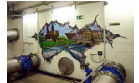
Pumping Station in IWB Lange Erlen
