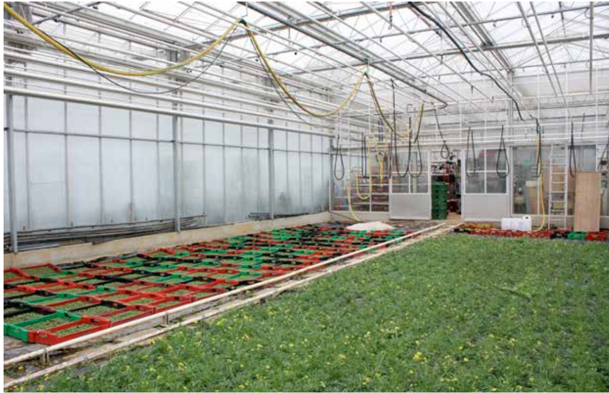
Greenhouse watering system at Birsmattehof/Therwil BL
