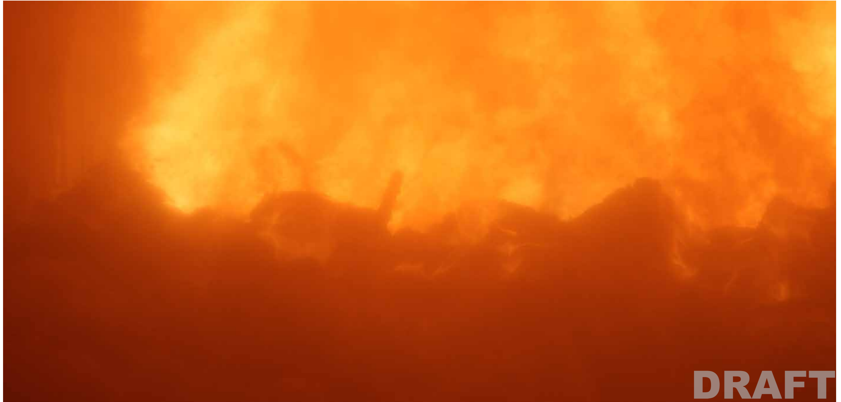
Combustion Chamber, KVA Basel
