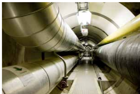
(9) hot water production
