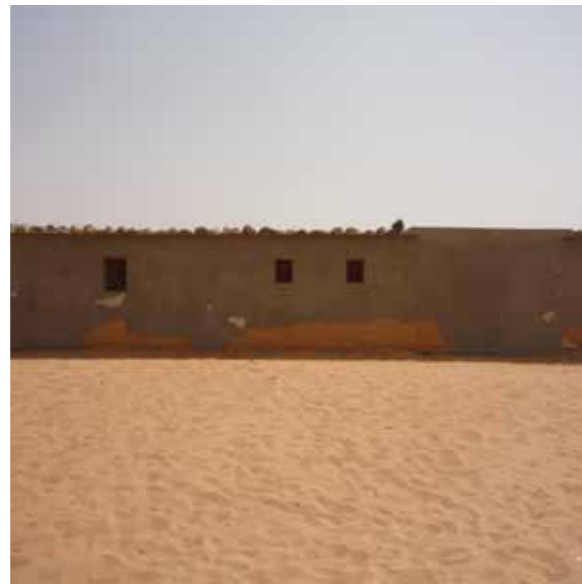
The cement plaster dropping off
