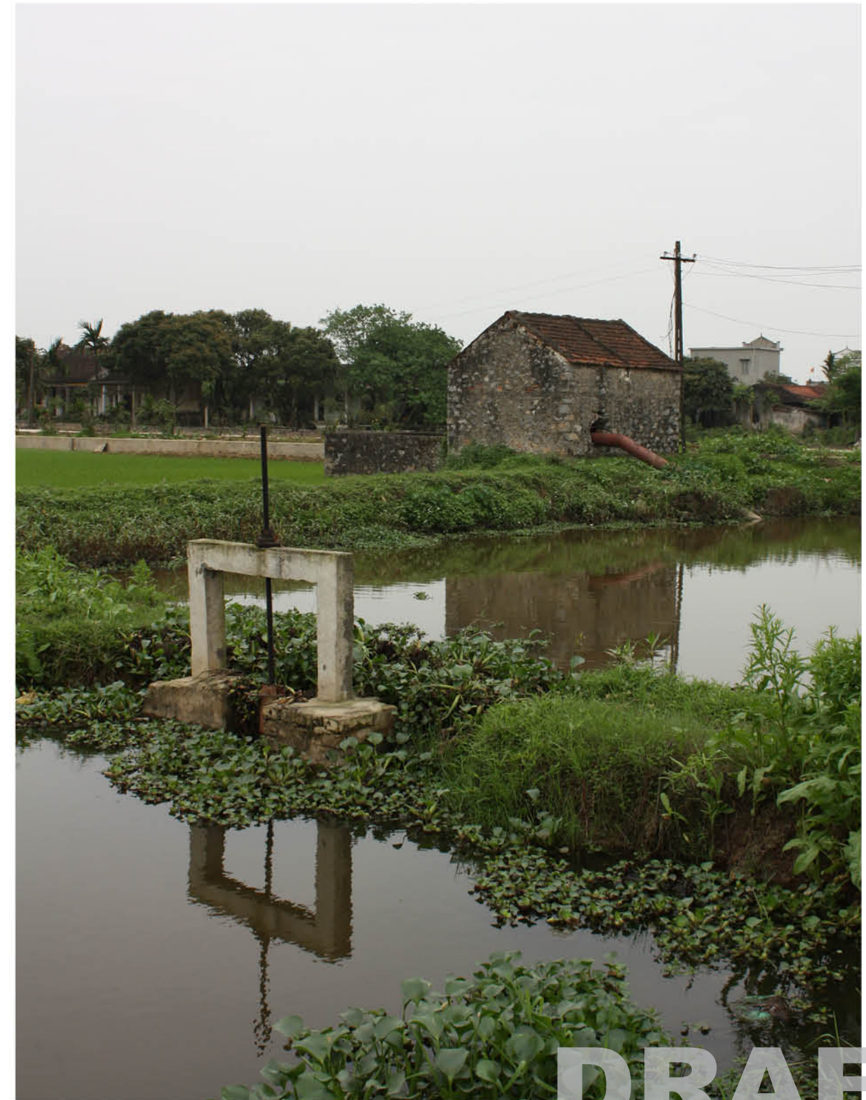
Pumping station Den To in Mai Son commune - Ninh Binh province
