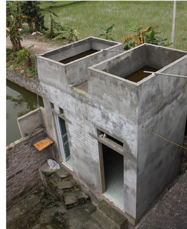
Rainwater collecting system
