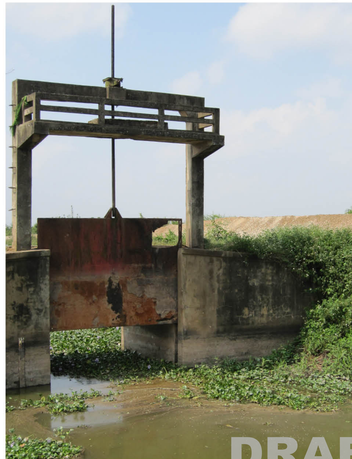
Outdated sluice - Nam Dinh province
